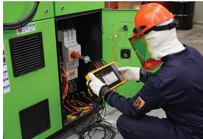
A Fluke 1777 Three-Phase Power Quality Analyzer in use. Power quality analyzers are one of the necessary types of tools for troubleshooting power quality problems.
